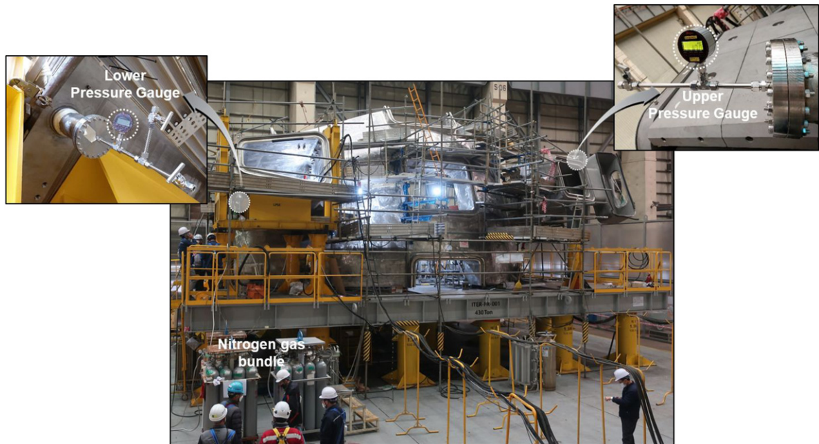
Figure 5. The picture of the actual installation of the pneumatic pressure test system. The lower pressure gauge is installed on the LPSE side, and the upper-pressure gauge is installed on the UPSE side. A bundle of five-nine purity nitrogen gas is connected to the LPSE connection.
